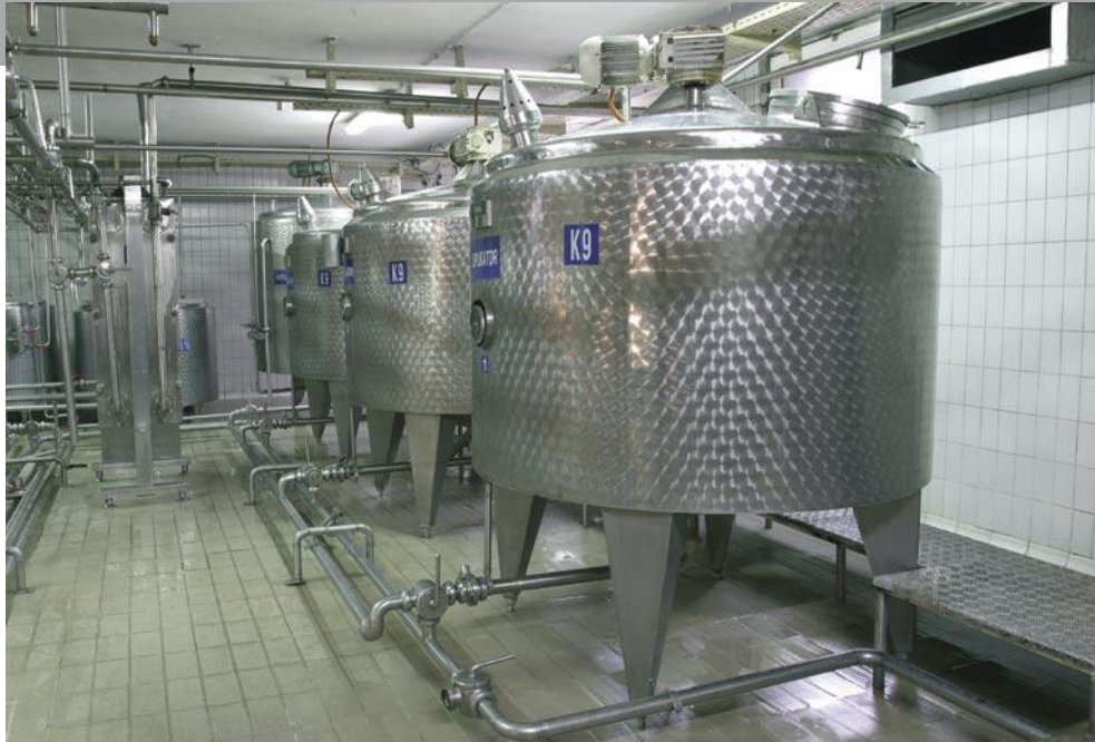
Secret mixtures of liquids are critical for the success of many food and pharmaceutical businesses. LABOM pressure transmitters play a key role in the accurate measurement of these valuable volumes of concentrates.
